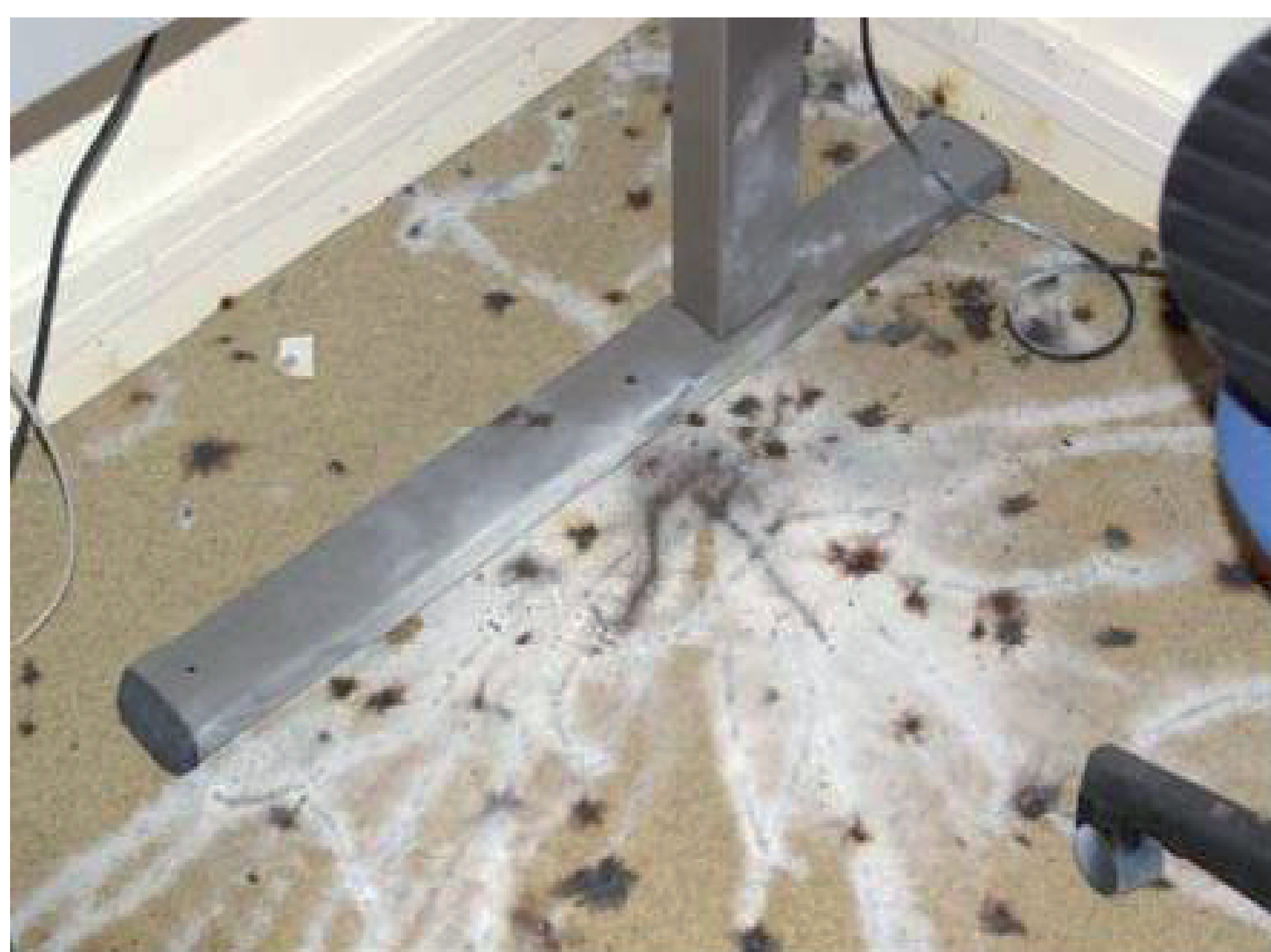
A typical ignition source has been found to be molotov cocktails or flammable liquids that are thrown into the school buildings. In this case the fire did not spread to other items.
